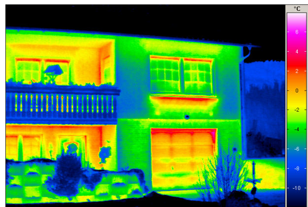
Heat loss below the window and at the door of the garage
