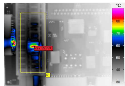
Img. 2: 5x digital zoom of thermal image of fuse block
