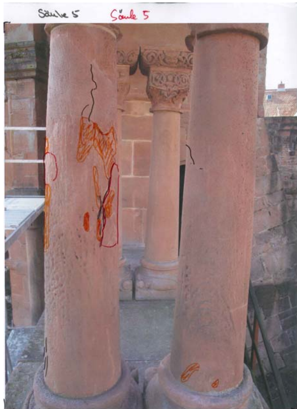
Figure 4: Pillar 5 (left), previous damage mapping, suspicion of subsurface detachment areas.
